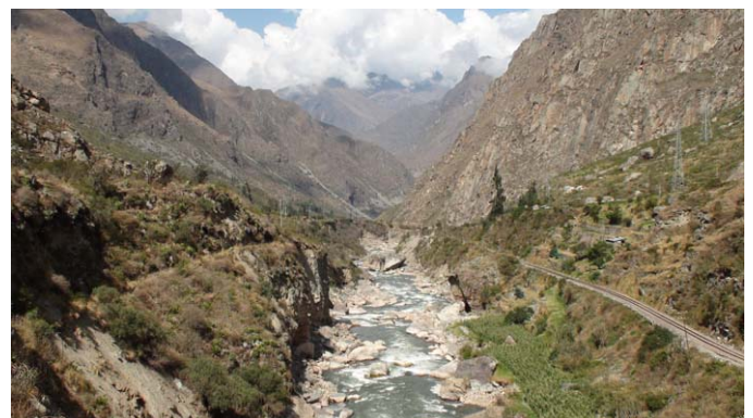
Looking down the Rio Urubamba in the direction of Machu Picchu. The sides of the river bank have been severely damaged in the recent floods.
